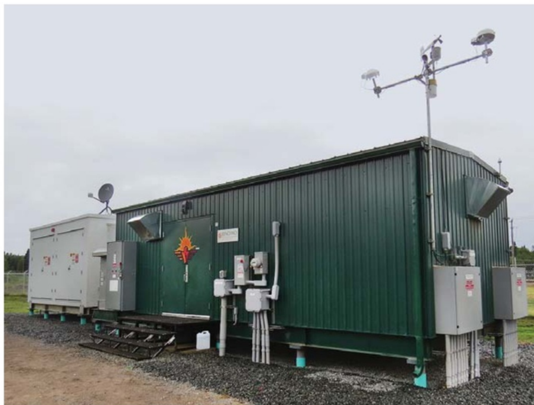
Outbuilding housing power equipment. The microgrid uses solar power, battery storage, and grid technology and supplies half of the community's energy needs, replacing the 130,000 liters of diesel fuel per year that the community was dependent on.
