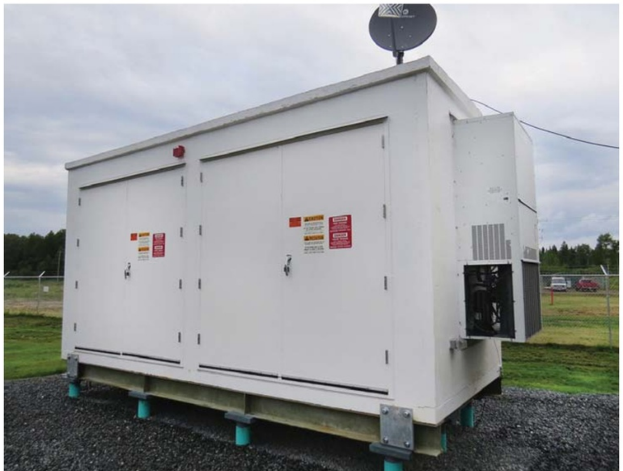
Battery energy storage building.
